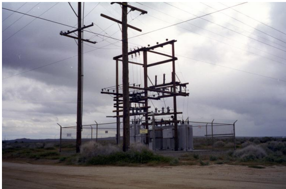
SCE North Muroc Sub-Station
