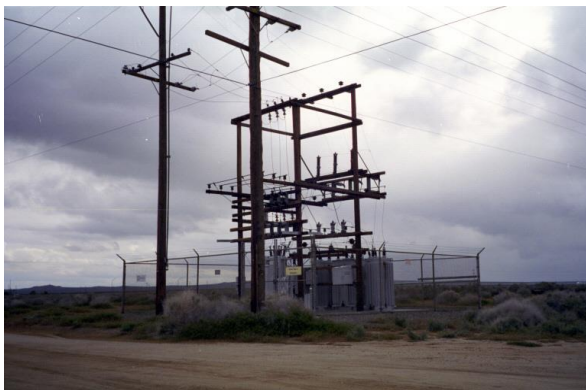
SCE North Muroc Sub-Station
