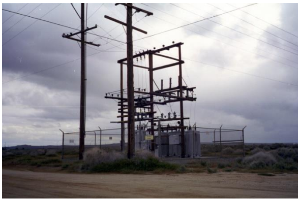
SCE North Muroc Sub-Station
